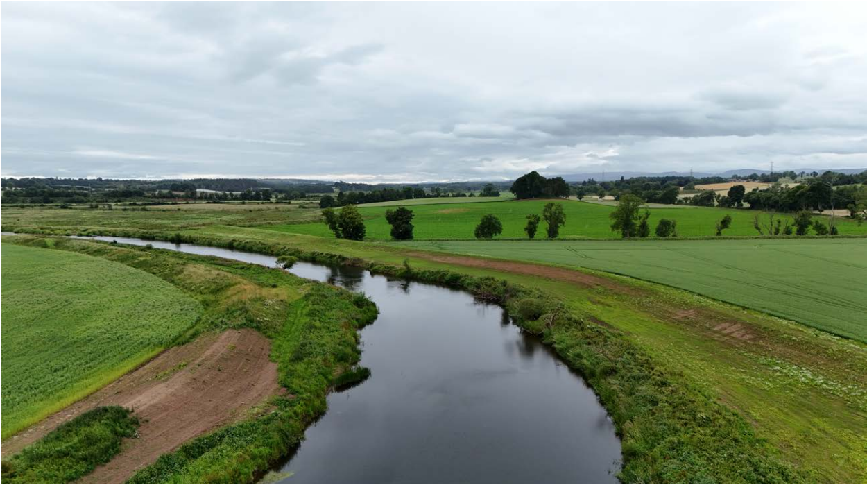
Aerial view of repaired embankments built in 2024 on the River Isla at Bendochy
